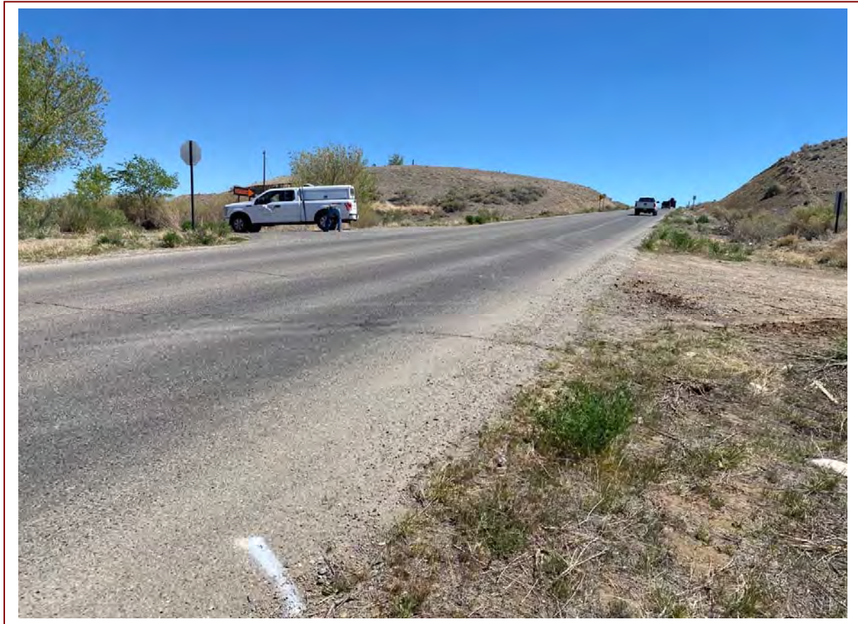
View of the site at Intersection of Bluff road and 36 taken on 4-26-21.
