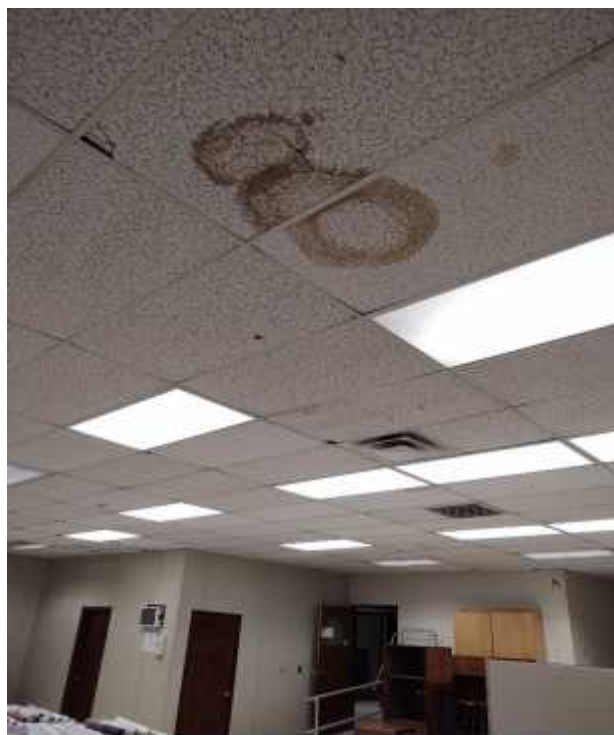
Multi Ceiling area have water damages from prior water leaks
