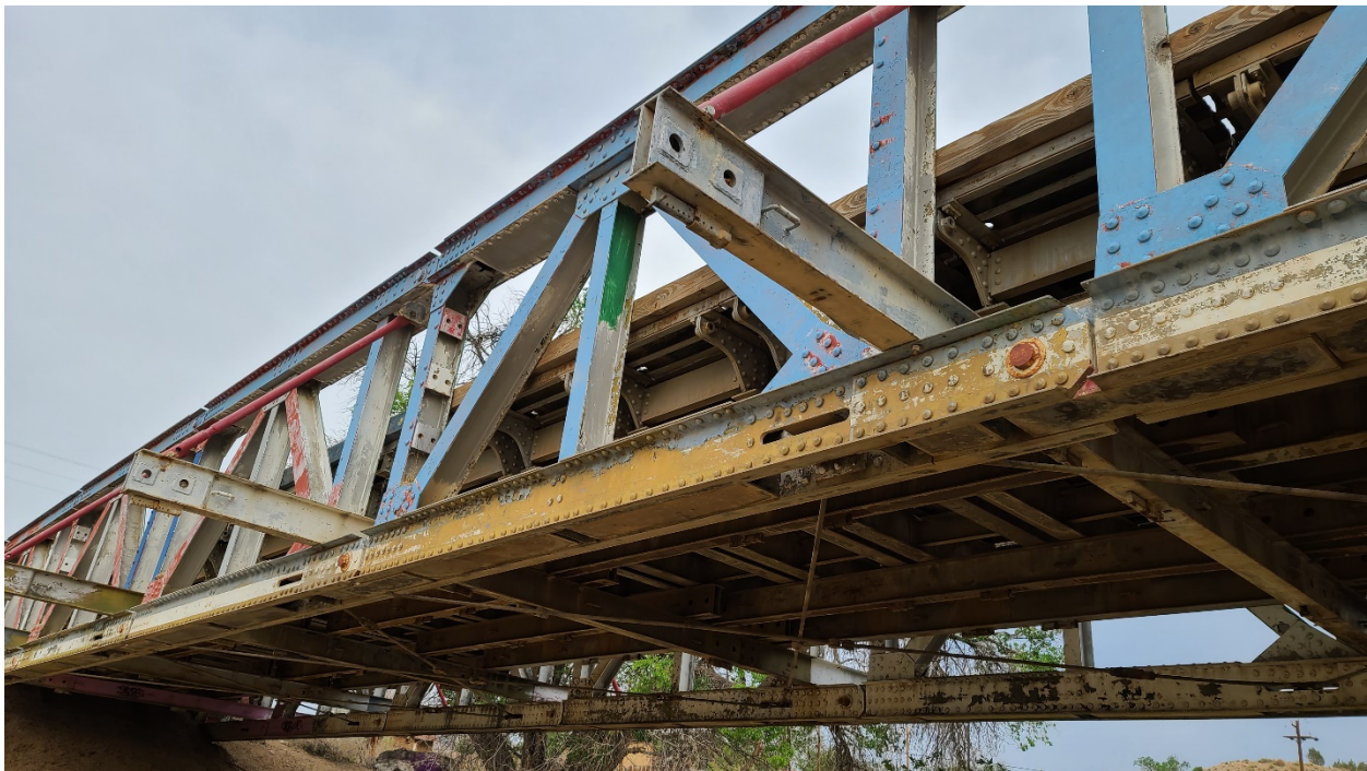
East side showing paint flaking off.
