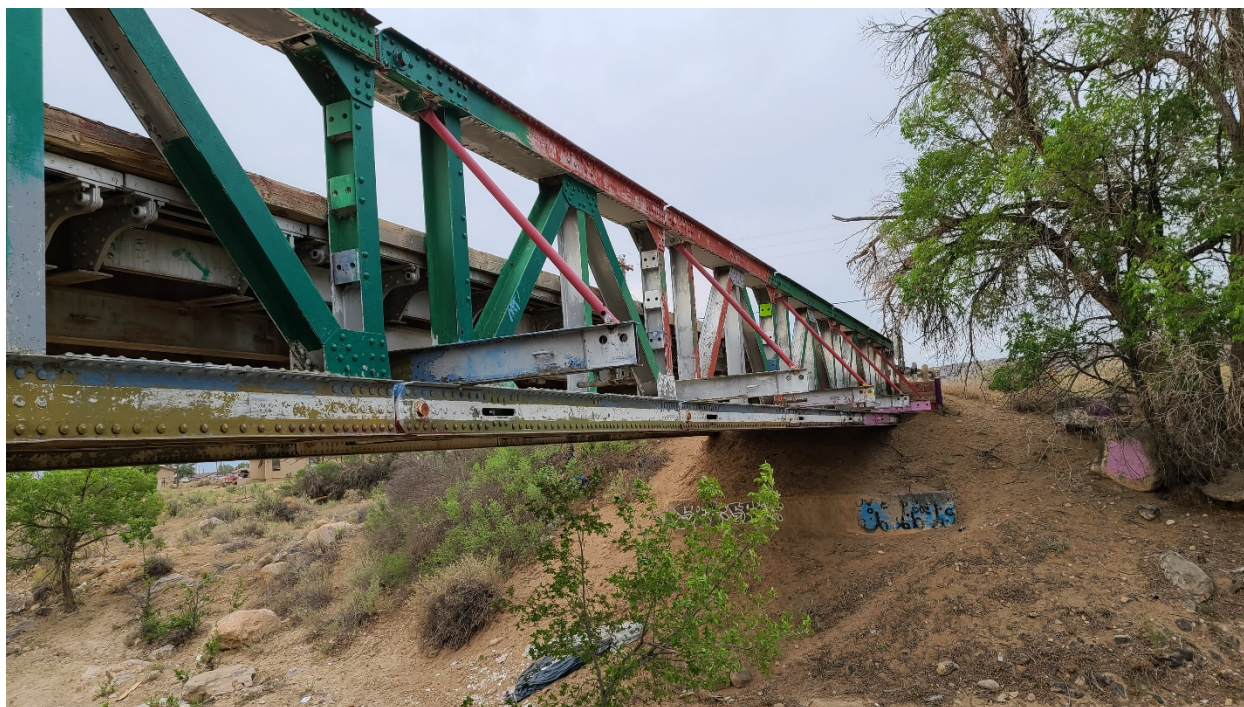
West side showing paint flaking off.
