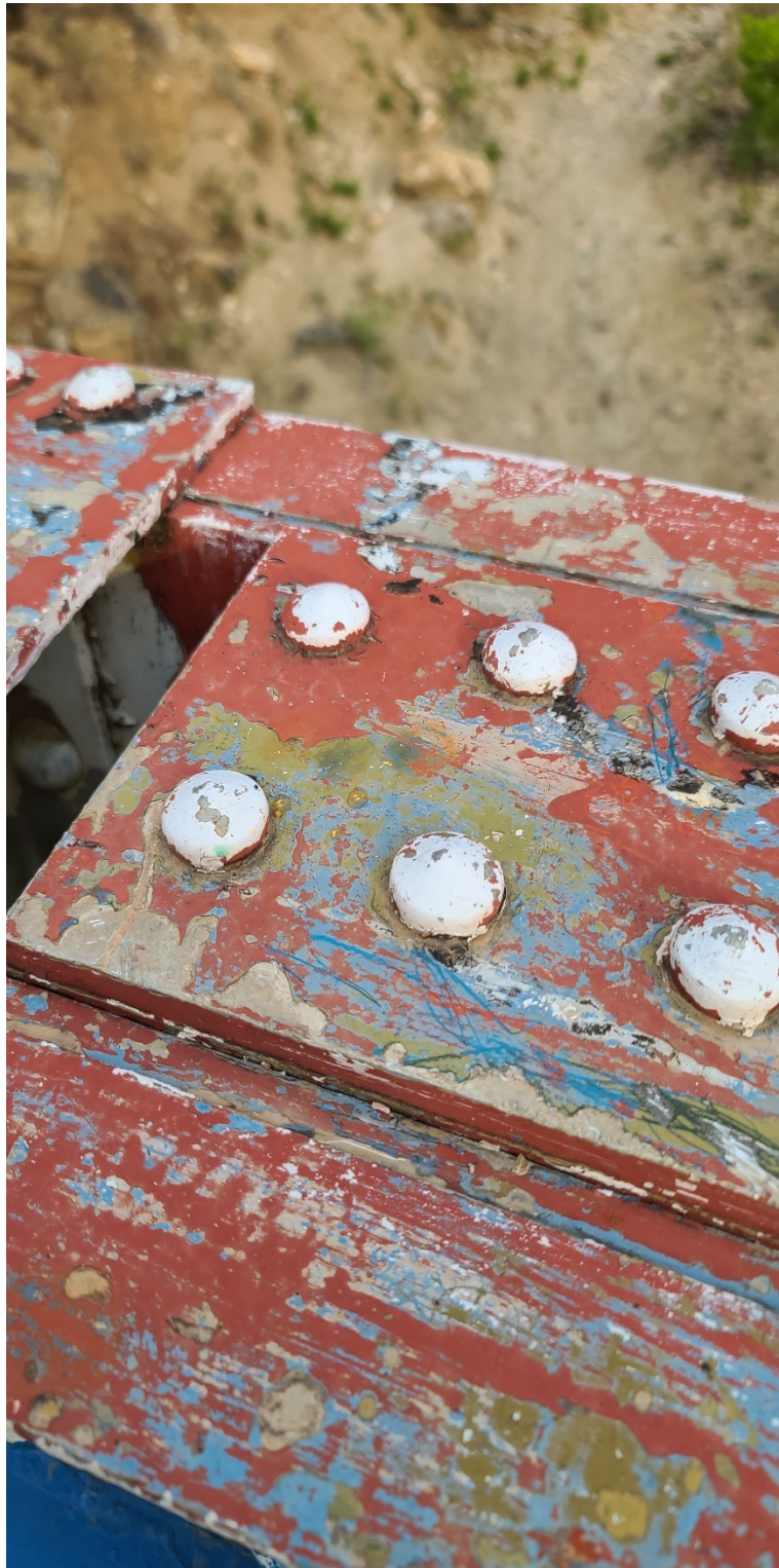
West Rail Red paint at mid span
