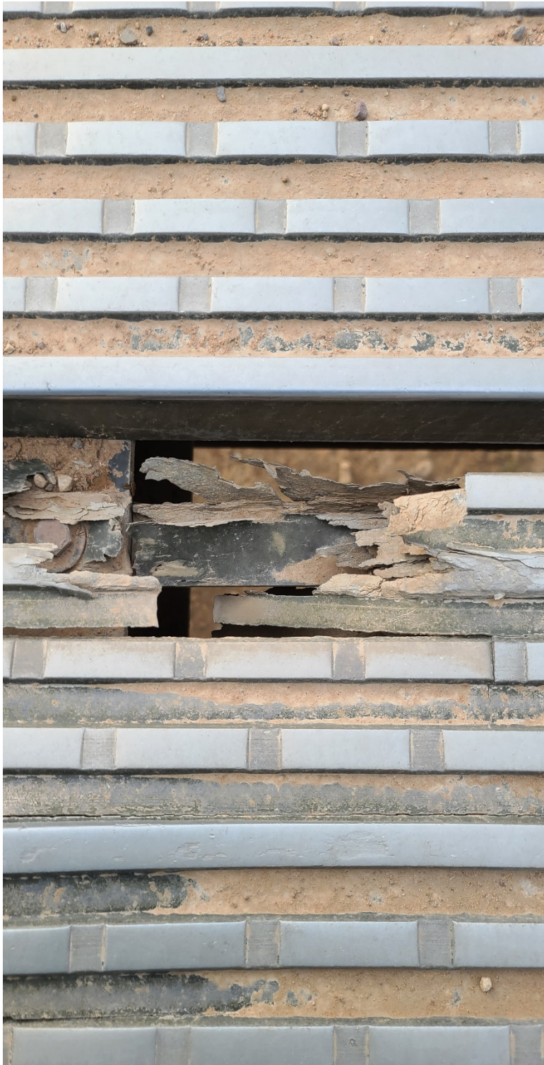
Bridge deck plates - damaged, with interior material degrading
